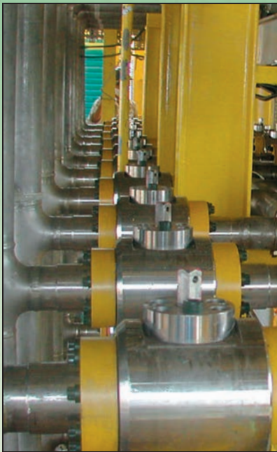
Manifold assembly prepared for actuator installation.
